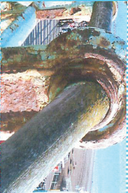
Seafront Railings Abandoned
